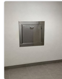
Bldg 10 Floor 2 Trash Chute Clear Sep 27, 7:18 PM CDT
