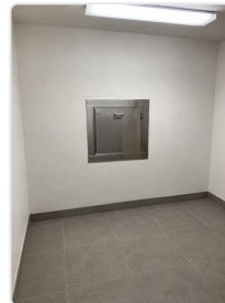
Bldg 10 Floor 2 Trash Chute Clear Sep 27, 7:18 PM CDT
