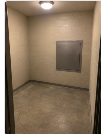
Bldg 11 Floor 2 Trash Chute Clear Sep 27, 8:08 PM CDT
